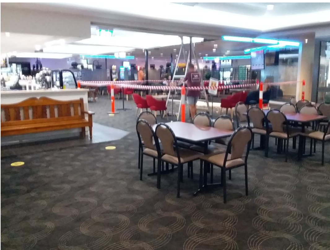
Ceiling collapsed in the club whilst we were having lunch.
